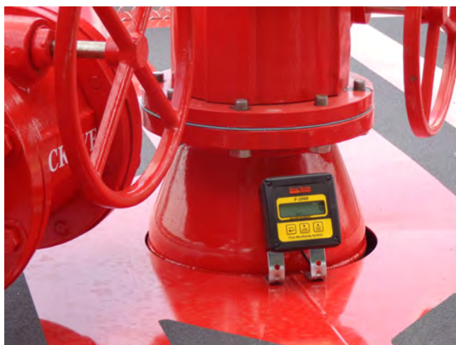
The monitor is provided with a pressure gauge and digital flow-meter to indicate actual flow through the monitor.
